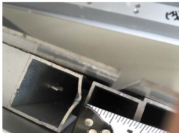
Photo 2: A damaged joint of the wall panel system.
